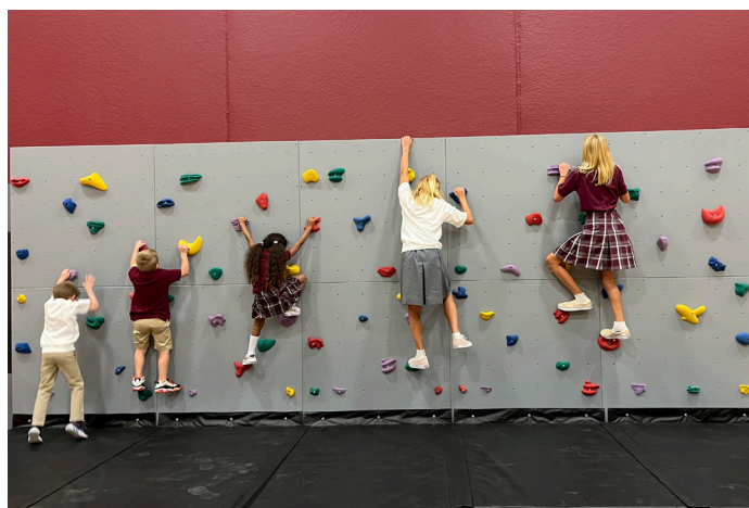
School of Grammar and School of Logic students tested out the new bouldering wall after its installation.
